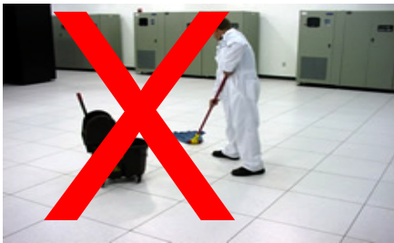
Improper Top-Floor Cleaning: Intro Of Water On Raised Floor
