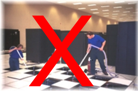
Improper Sub-Floor Cleaning: Creating Bypass Air Flow
